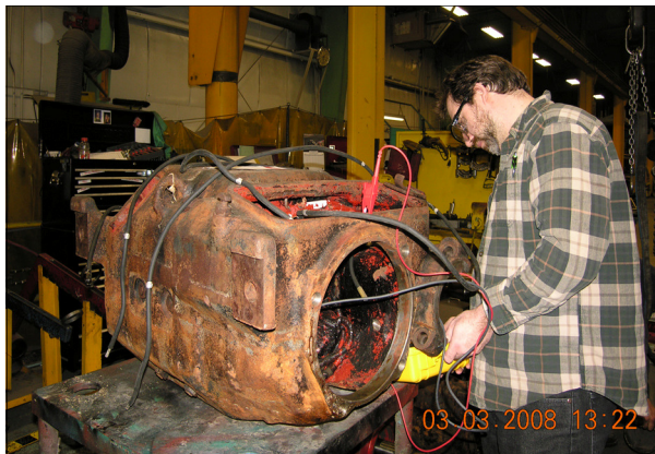
Seashore's Restoration Technician Randy Leclair at A. C., measuring the insulation resistance of one of 1227's motors
