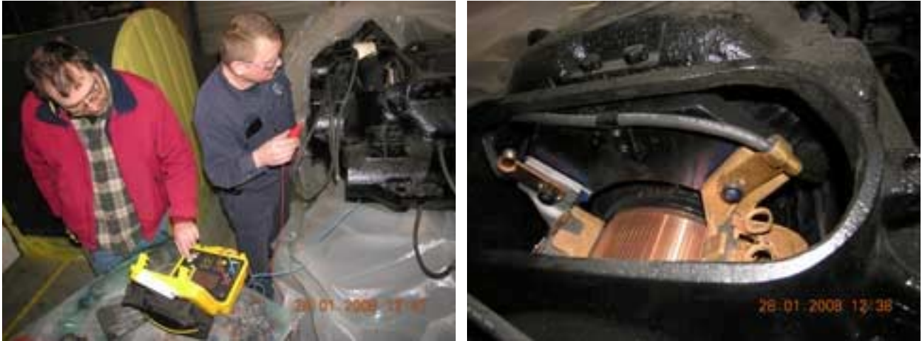
Randy Leclair monitoring the new AEMC 1060 megohmmeter while Roger Paradie makes the connection to the overhauled GE 80 motor at A. C. Electric
