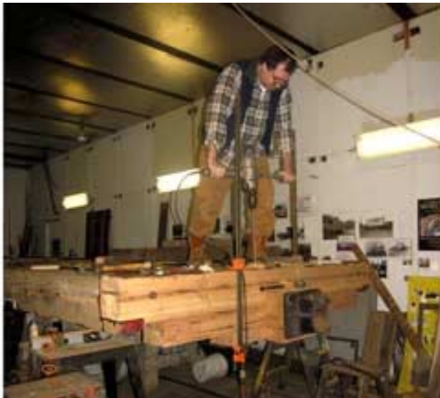
Randy Leclair using the big drill to make holes for bolts to fasten sill assembly together.
